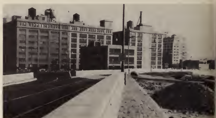
A granite wall separates the north and south roadways, the north roadway shown completed and ready for traffic.
